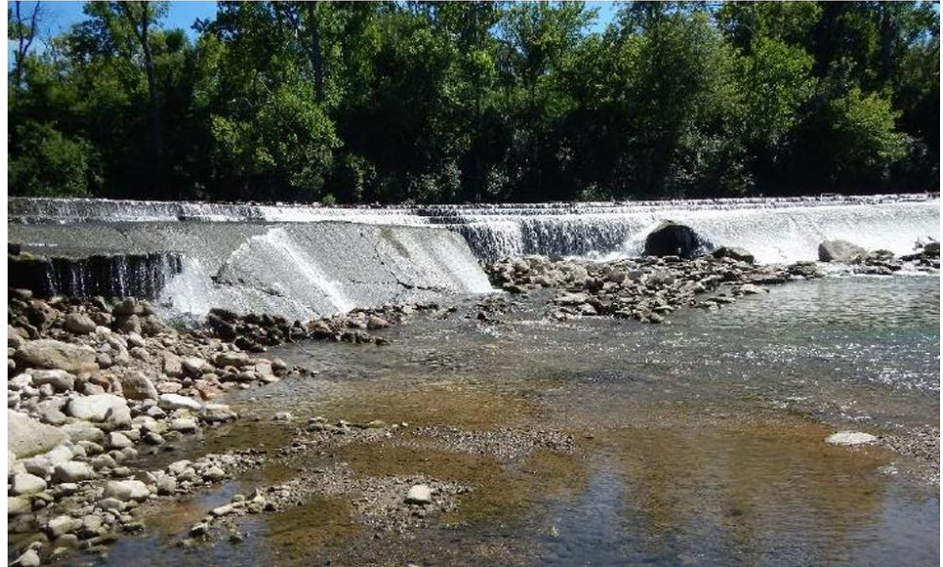
Photo of existing dam, showing broken portion of dam (Credit: Ohio EPA Preliminary Finding of No Significant Impact and Environmental Assessment)
